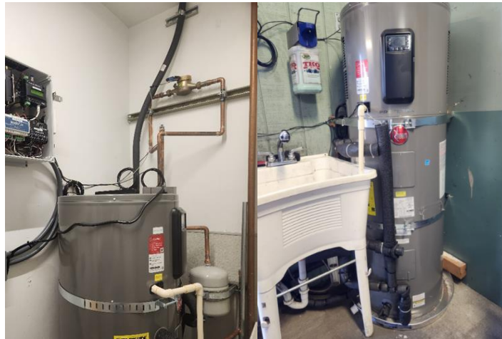
Figure 6. 120V HPWH installation at demonstration site 1 (left) and 2 (right). Source: EPRI
